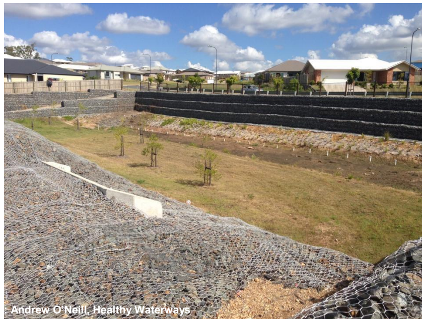
Figure 1 Example of a poorly designed bioretention basin with high retaining walls and steep batters
